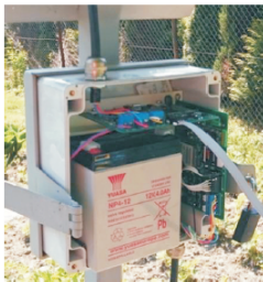
Main station (interior)
