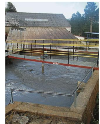
Lime conditioner of the mine drainage
